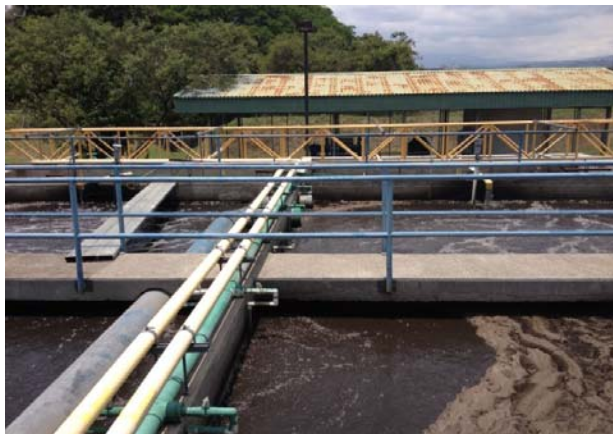
Figure 49: Waste water treatment plant. Source: Picture taken during onsite visit, April 2013
