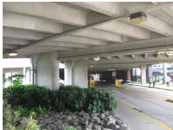
Figure 34: Change of the parking lights with LED ones Source: Picture provided by AERIS, April 2013
