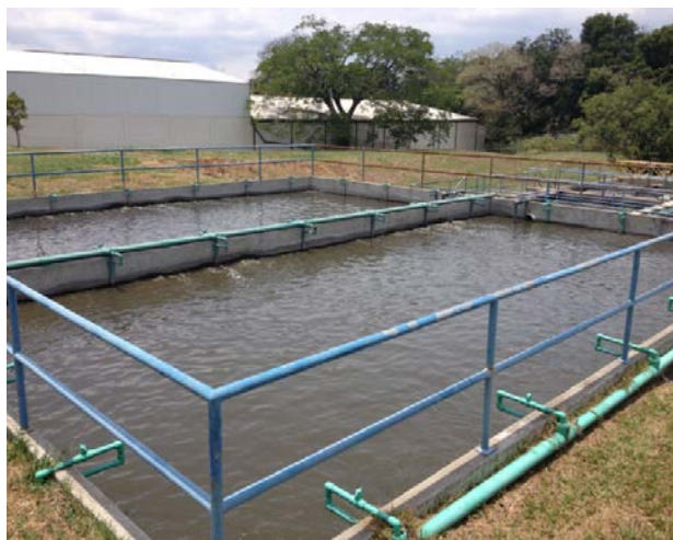
Figure 17: Water treatment plant.
