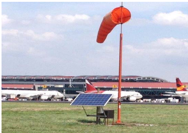
Figure 33: Use of solar energy to provide power to the meteorological station. Source: Picture provided by AERIS April 2013
