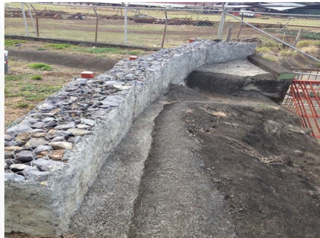
Figure 56: Measures to prevent overflows. Source: Picture taken during onsite visit, April 2013
