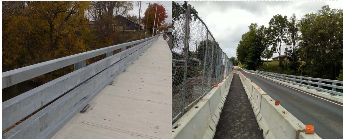
Fig.28: Open steel railings for better integration to the surroundings
