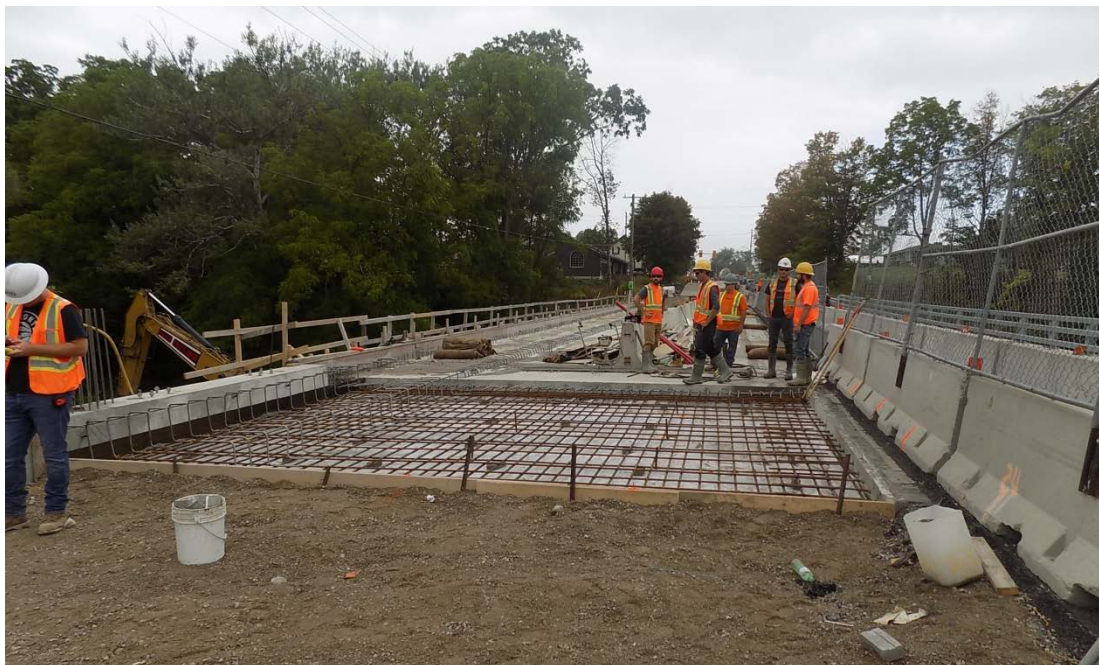
Fig.22: Use of Duplex 2205 grade stainless steel in the entire deck and approach slabs
