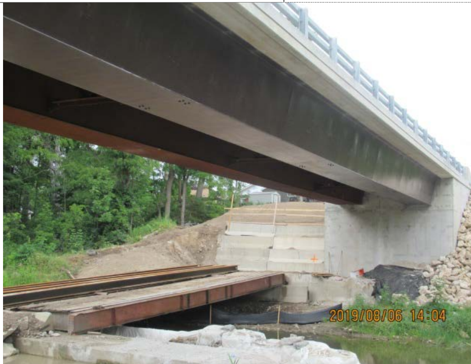
Fig.30: Metalized coating on the exterior and bottom face of the exterior girders
