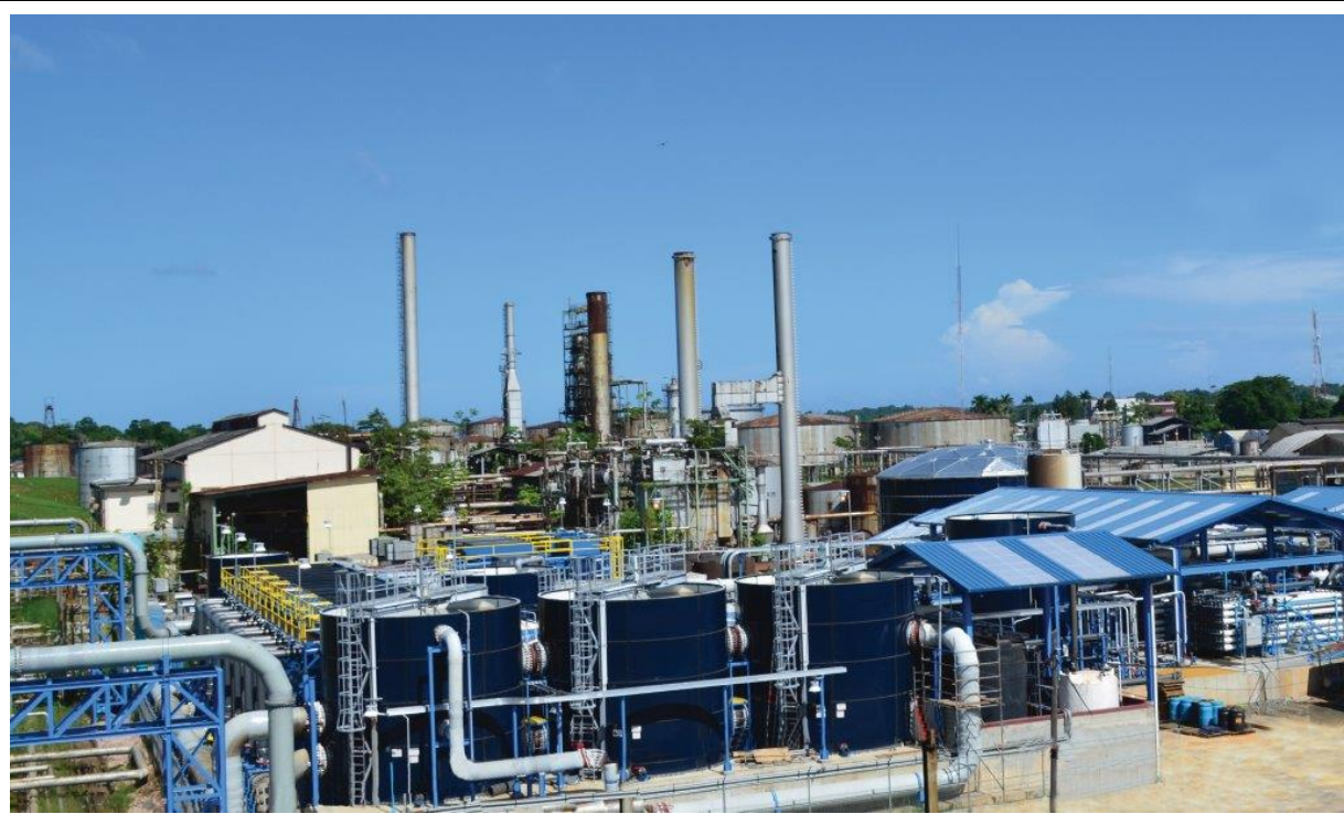
Figure 1: Point Fortin Desalination Plant Sources: Seven Seas Water Company Images
